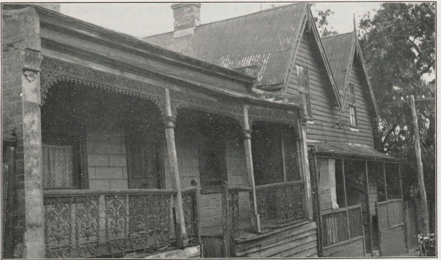
A house typical of the state of disrepair into which many dwellings have been allowed to fall. This one has been renovated since the Board's inspection.
