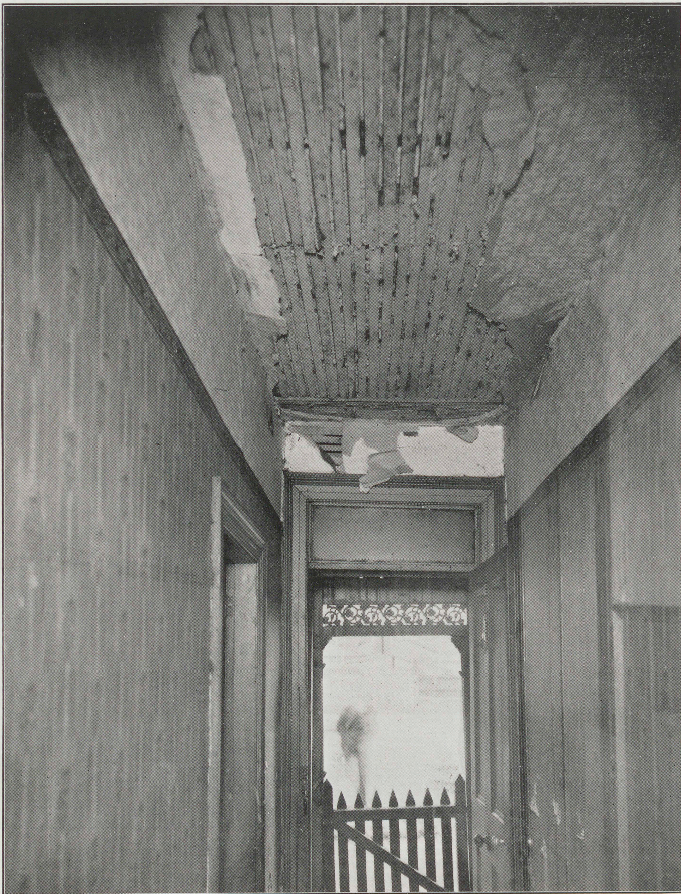
A defective ceiling illustrated. Large pieces of plaster fall regularly and are a constant menace to the occupants.
