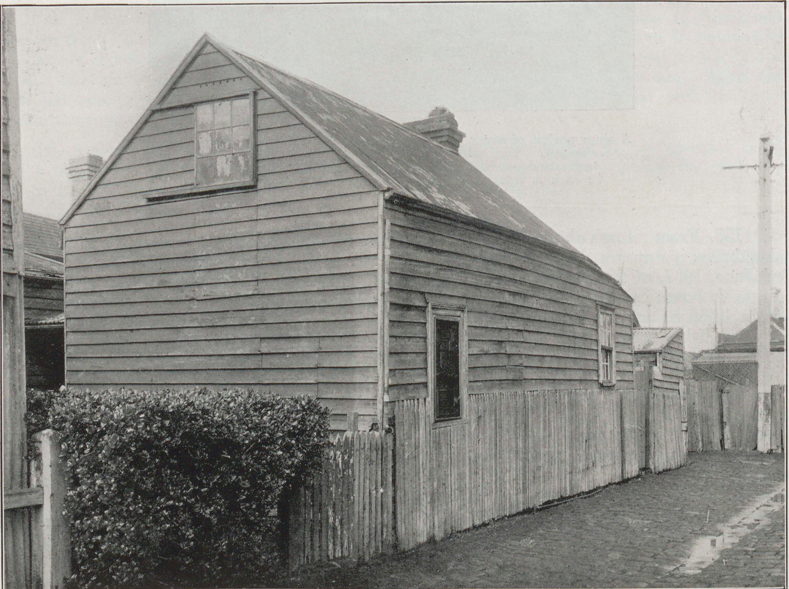
One of three dwellings in Palmerston-place, South Melbourne. Rental 12s. per week. Its external appearance is a guide to its general condition.
