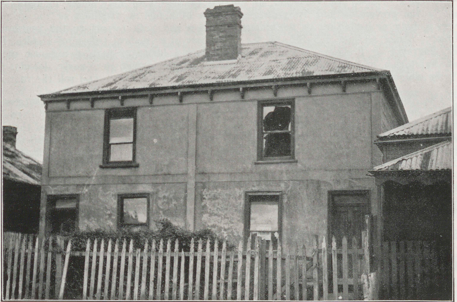
The above dwelling was photographed in Williamstown. A "TO LET" notice is displayed in the window. As the outside appearance would suggest, the whole structure is in a dilapidated condition and illustrates the necessity for legislation for regular inspection of rented premises as recommended in paragraph 140, section 3.
