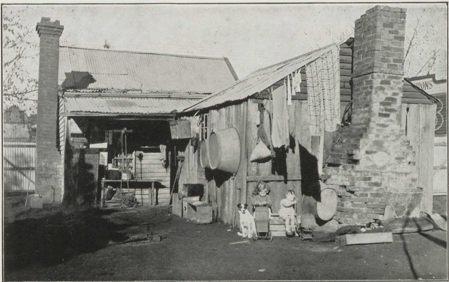
Rear of dilapidated house in Fryers-st. The house has been condemned, but tenants pay 12s. 6d. weekly in rent.
