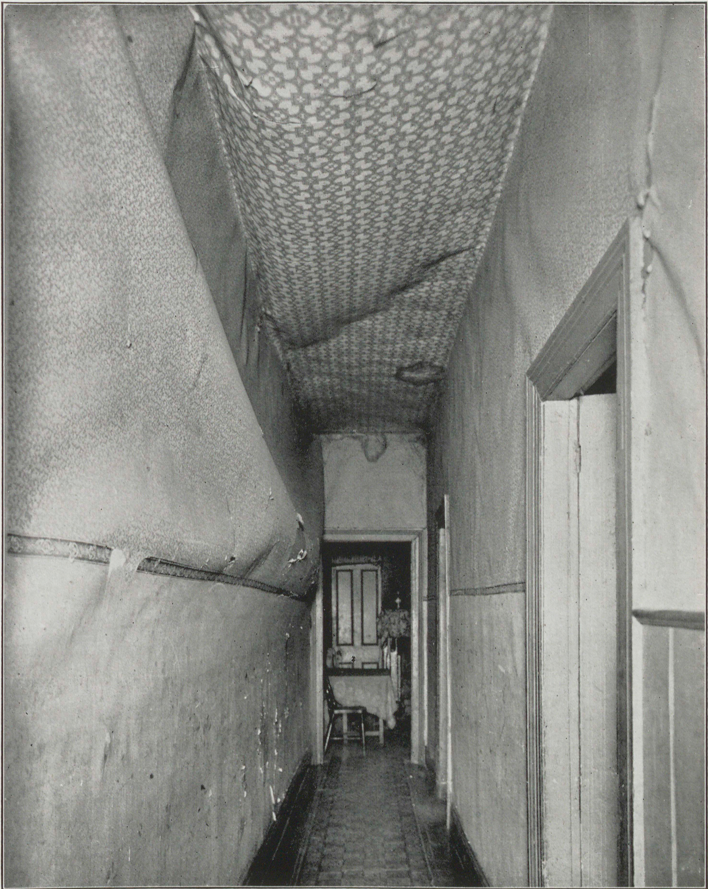
A party wall of timber frame and hessian and paper in a house in South Melbourne. The whole paper and hessian had become detached from the frame and bulged into the passage. The ceiling is in similar condition. Repeated requests for repairs to this house met no response.
