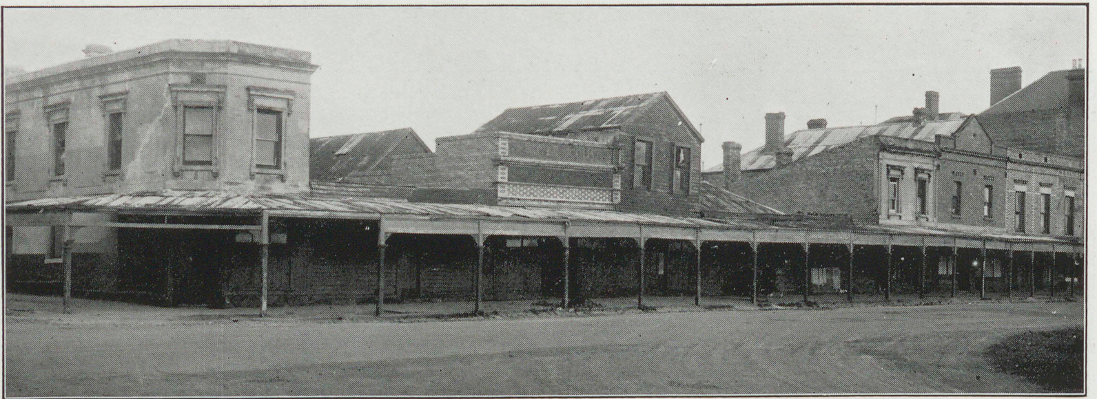
A row of old shop premises in Williamstown, some of which are now used as residences. They are totally unsuitable for occupation as dwellings, and recently the local municipal authority has condemned two of them.
