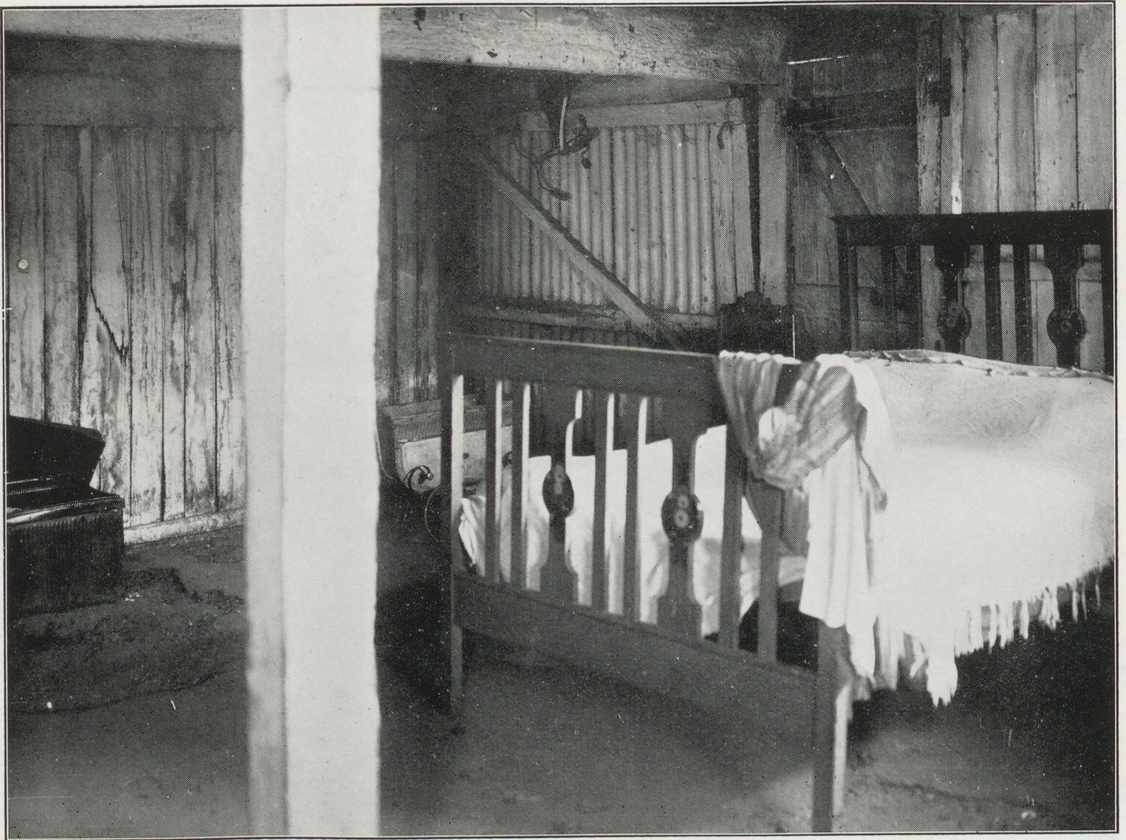
The bedroom of above factory residence. Holes one (1) square yard and more in area occur in many parts of the asphalt floor, which has no covering whatever.
